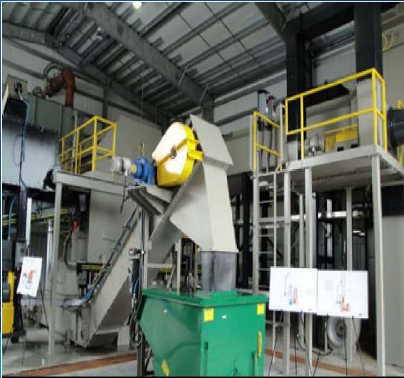
Municipal Sewer Sludge gasification plant, Sanford, Florida (USA)
