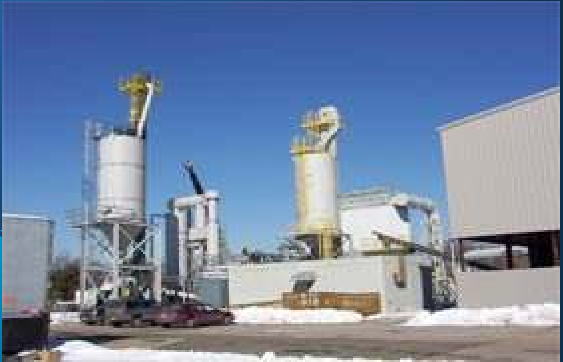
Municipal Sewer Sludge gasification plant, Philadelphia, Pennsylvania (USA)
